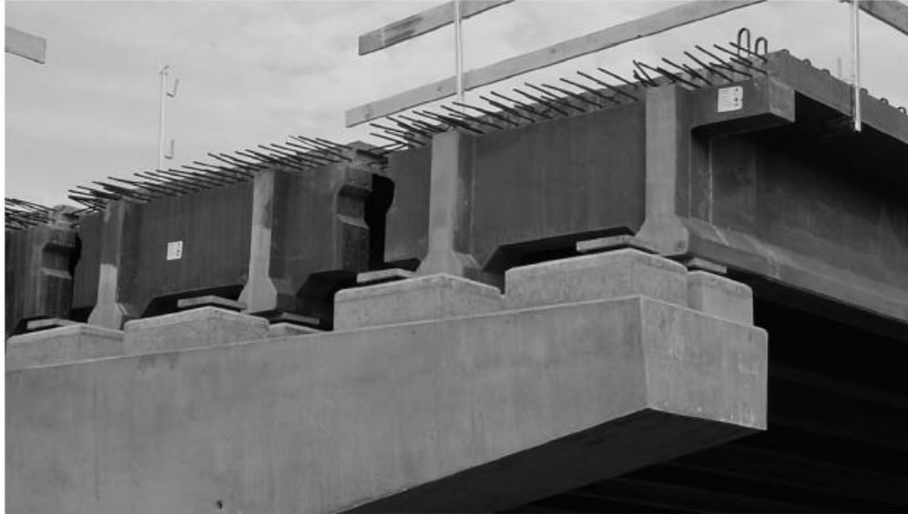
Figure 3: Road Bridge at Bourg-les-Valences. Central pier during placing of pi-shaped beams (Vergoossen, 2008)
