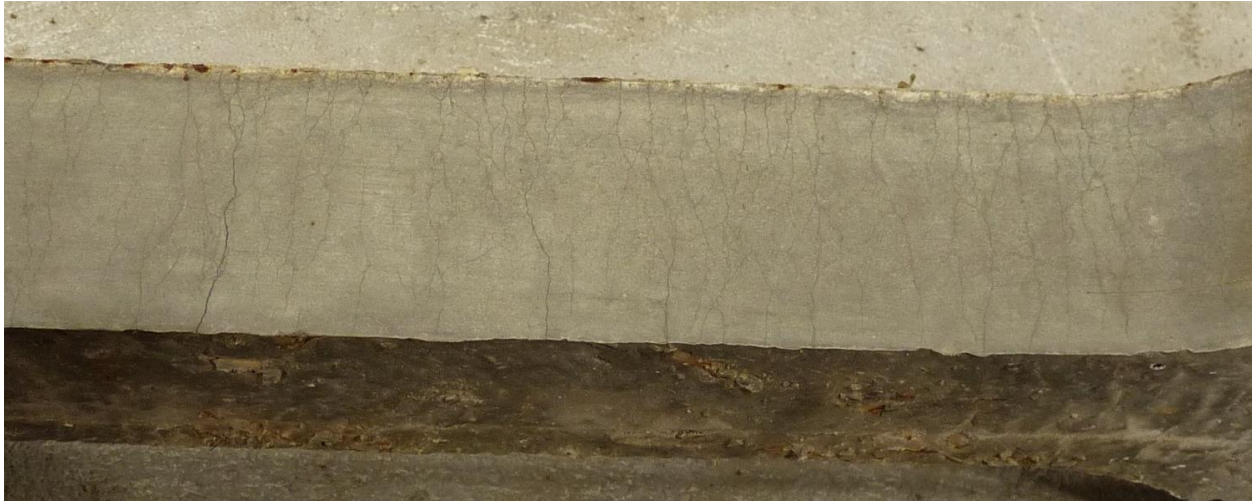
Figure 46: Micro-cracking in Supplier 1 - 2% Fiber Specimen
